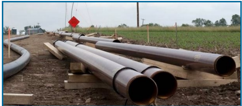
Coudersport photographer Curt Weinhold provided this picture of a Tioga County setting where workers were preparing to install pipes to usher shale gas to market.
