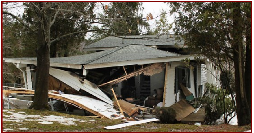
A house in McKean County was destroyed by a 2011 natural gas explosion. The gas migrated from a nearby well that was abandoned long ago.
